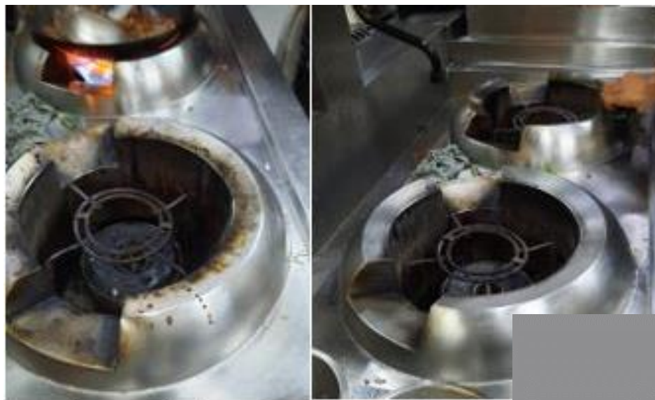
Before and after cleaning with Aqueous Ozone during service
